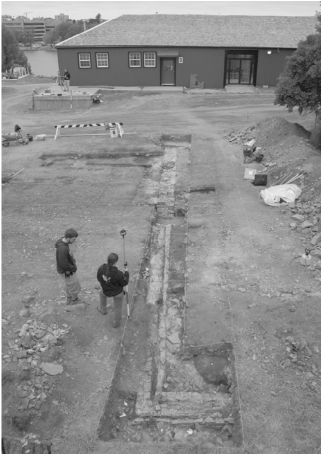
Figure 2. South foundation of the blacksmith shop looking west. Photo by J. Last (Parks Canada, Ontario Service Centre, ARD photo no. 131H1877E).
