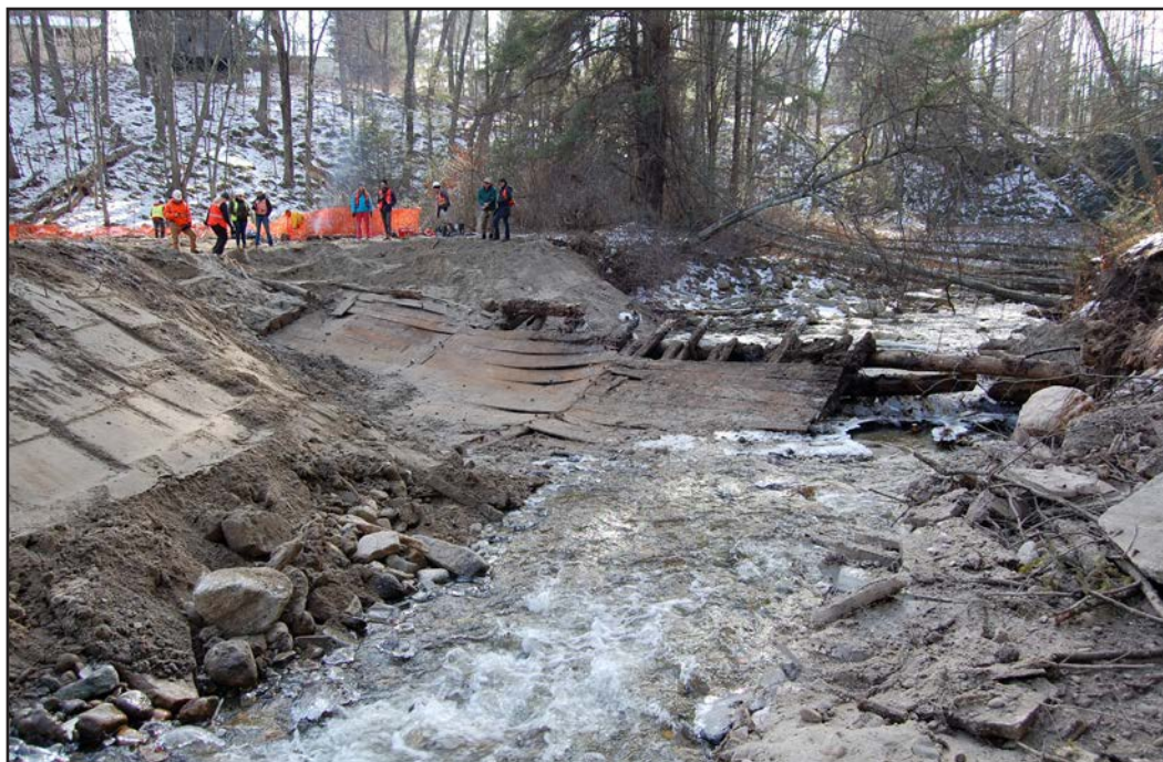
Figure 4. General view of fully excavated Timber Dam, north bank of brook looking southwest.
